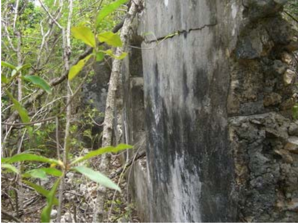
5. The ruined and overgrown, plastered inside wall of the curing house at Benzies (by the author).
