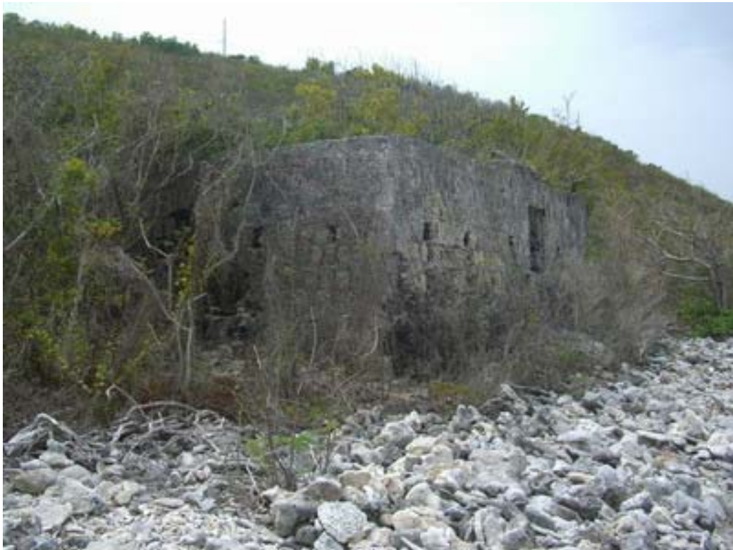
4. The overgrown ruin of the sugar boiling house at Benzies (by the author).
