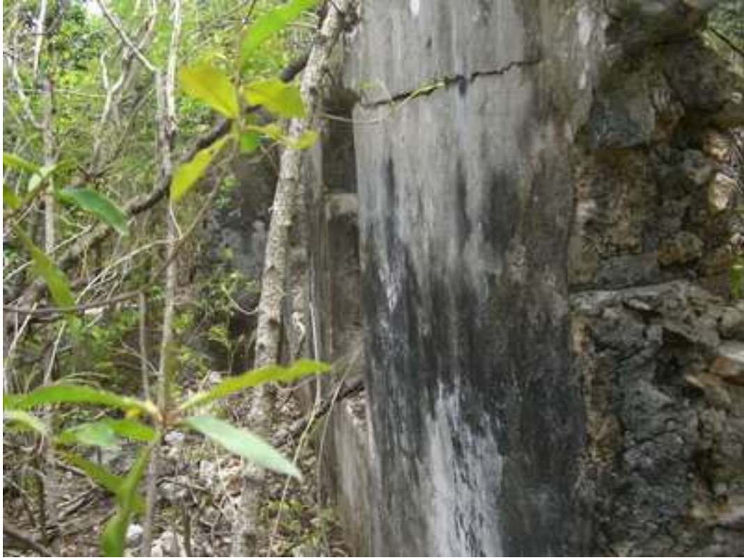
5. The ruined and overgrown, plastered inside wall of the curing house at Benzies (by the author).
